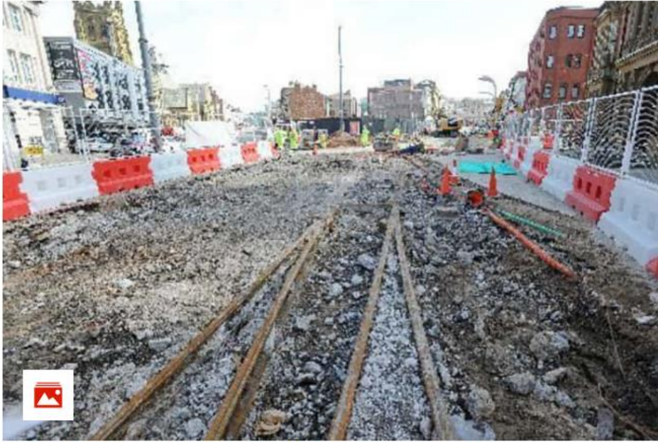
Tram tracks have been uncovered on Talbot Road outside the Town Hall
